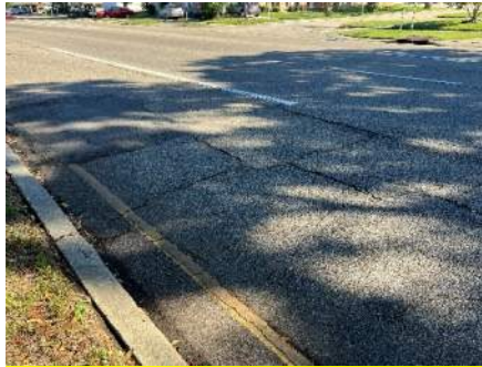
Figure 1: Existing Asphalt Deterioration
