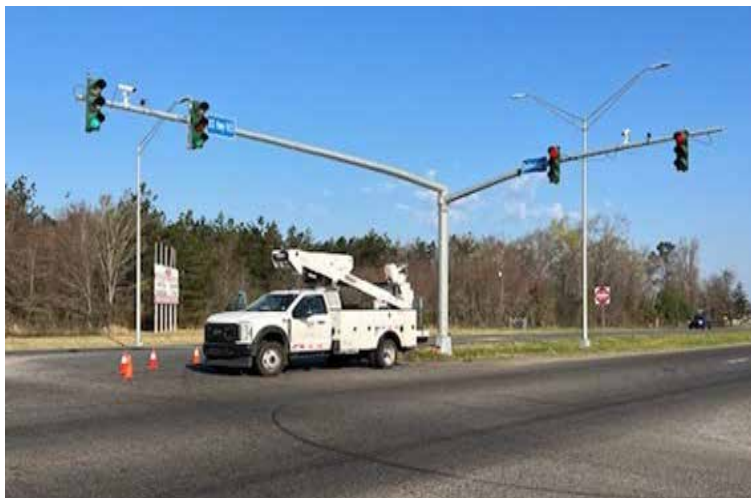
Radar installation on a signal along U.S. 80
