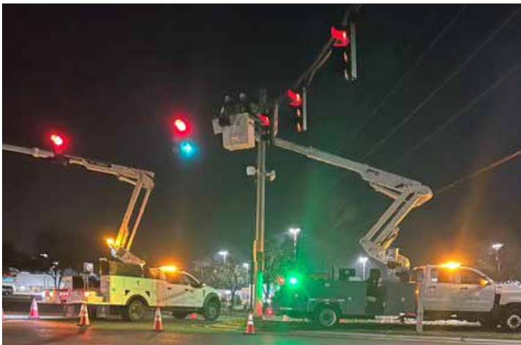
Radar detection equipment installation in St. Tammany Parish
