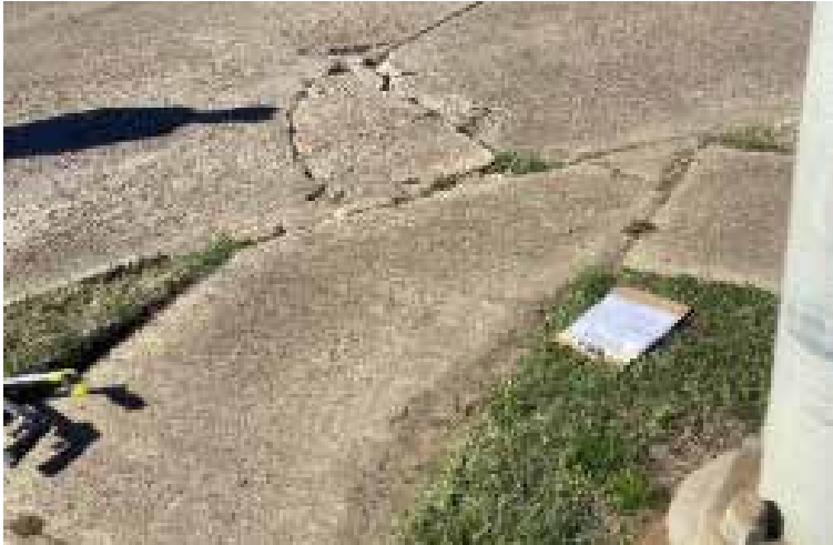
Area of LA 511 needing repairs in Caddo Parish
