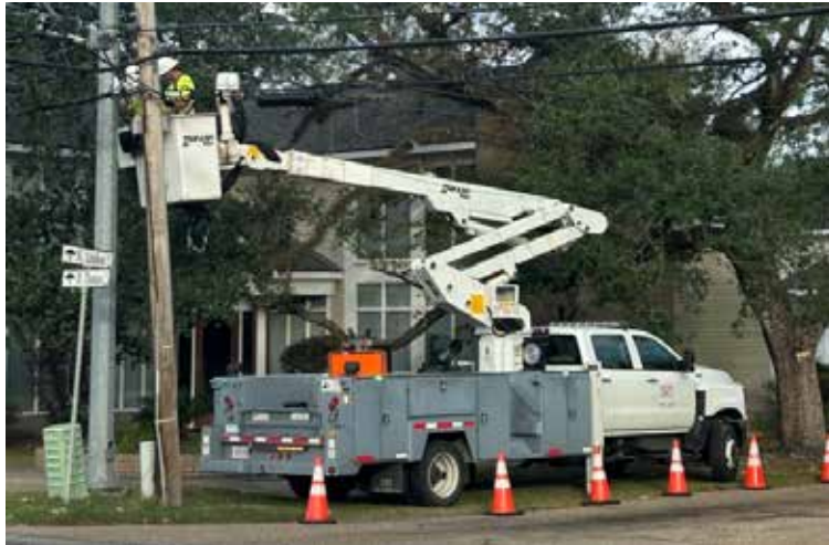
Installation of radar detection equipment
