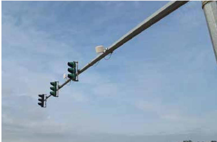
New radar detection equipment
