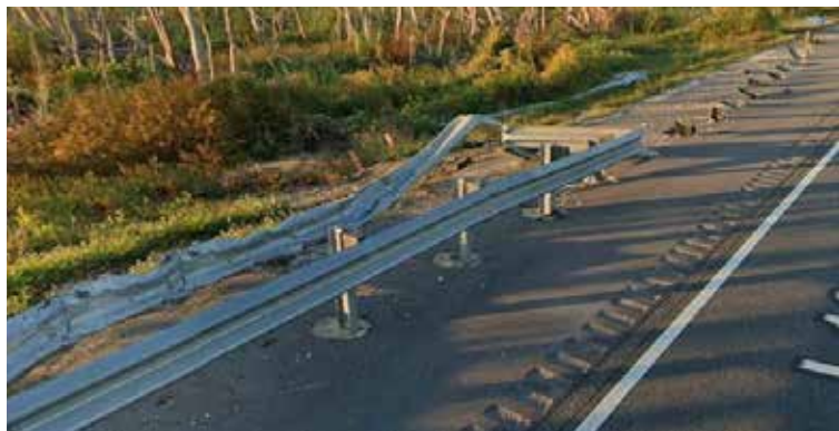
Guardrail damage on I-10 westbound near Michoud Boulevard
