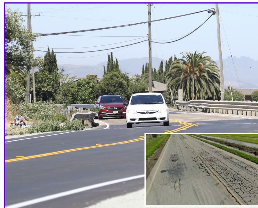
Inset photo shows the severely deteriorated condition of the pavement prior to TRC's design efforts for a full-depth reclamation and overlay.
