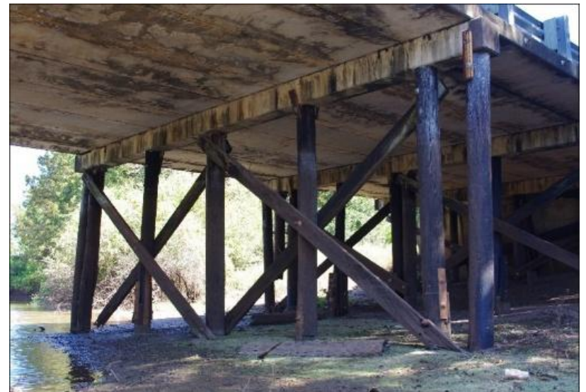
Deteriorated and Repaired Bent Inspected and Repaired by Forte and Tablada
