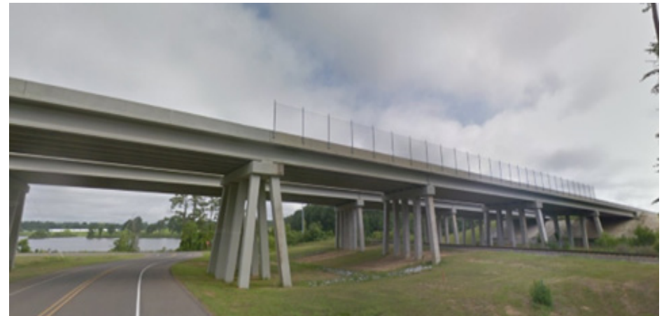
GEC provided design of the bridge over the KCS Railroad in Alexandria without impacting the railroad during construction.
