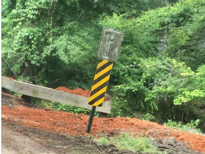
Figure 3-12: Illegible weight limit sign
