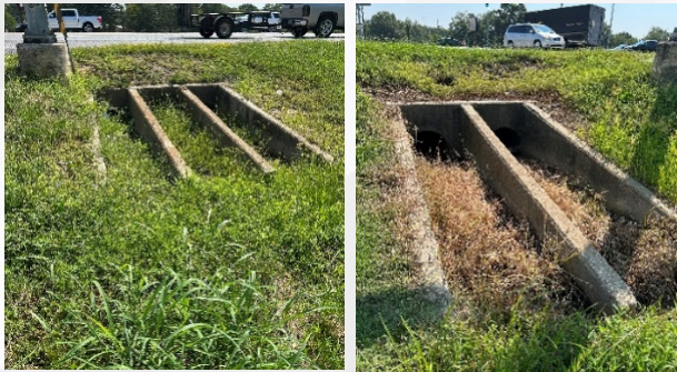
Figure 9: 18" drainage pipes at Louberta St.
