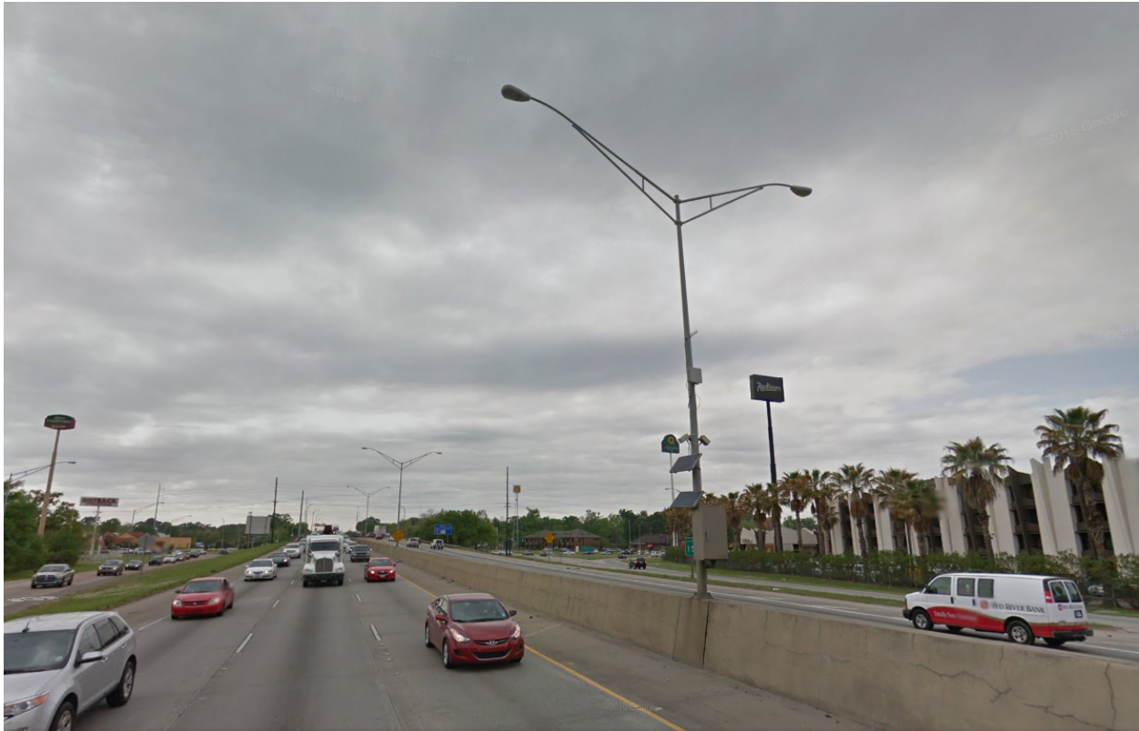
Figure 15: Vehicle Detection Systems Mounted on Lamp Post
