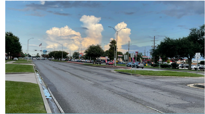
Existing Ponding on Roadway
