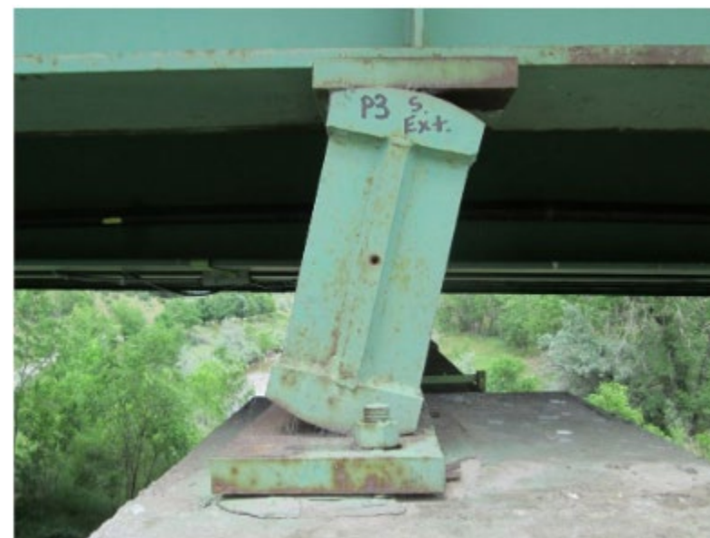
Existing bridge deficiency: Tilted girder bearings past critical angle
