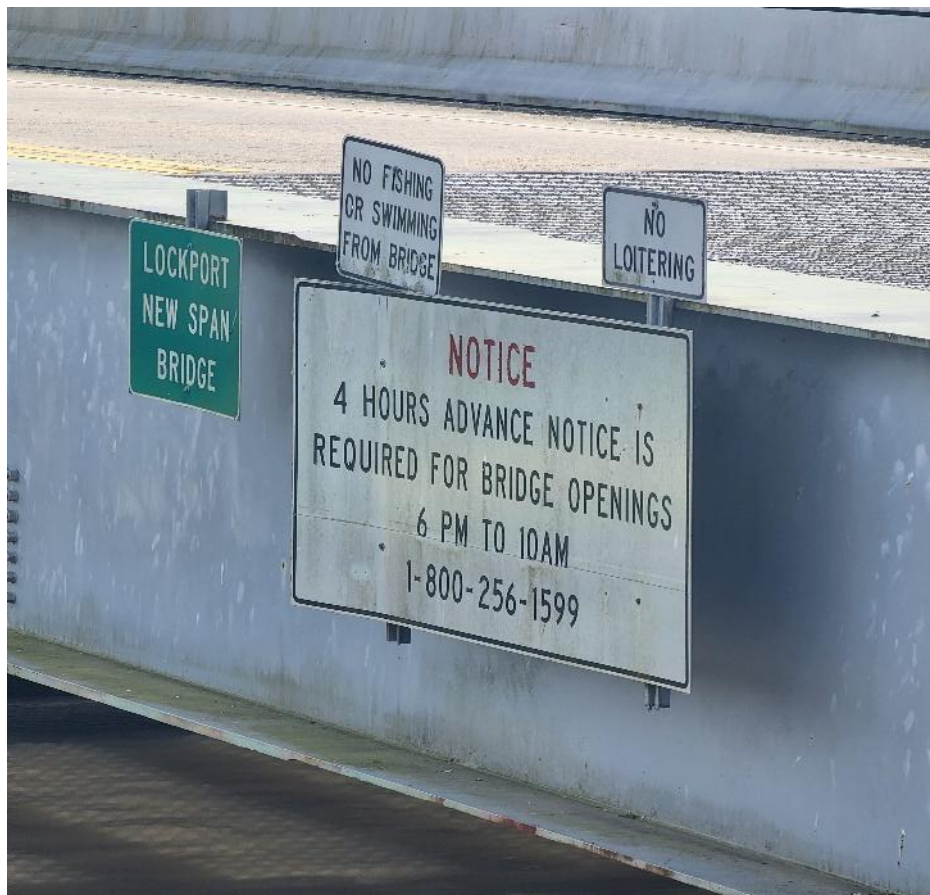
Figure 5-13: Signage attached to hydraulic swing bridge.
