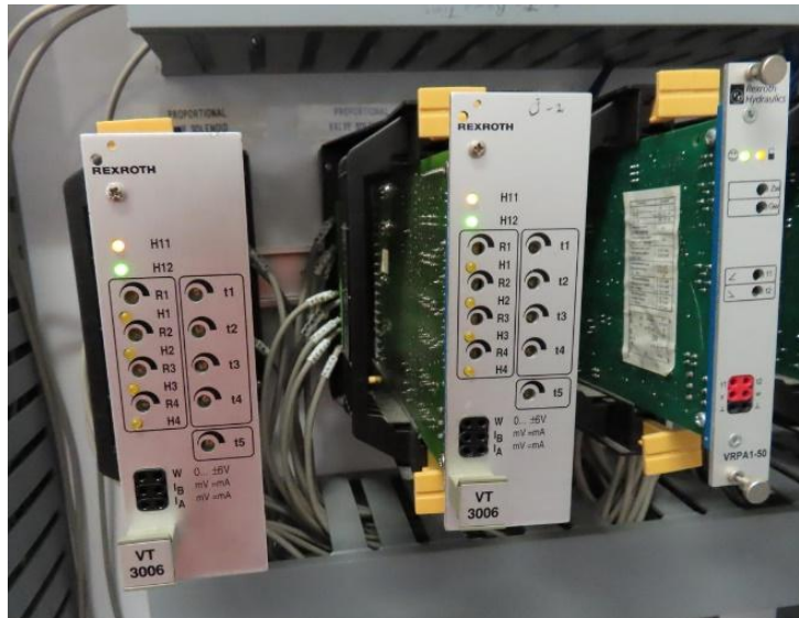
Figure 4-63: Amplifier Cards in a cabinet.
