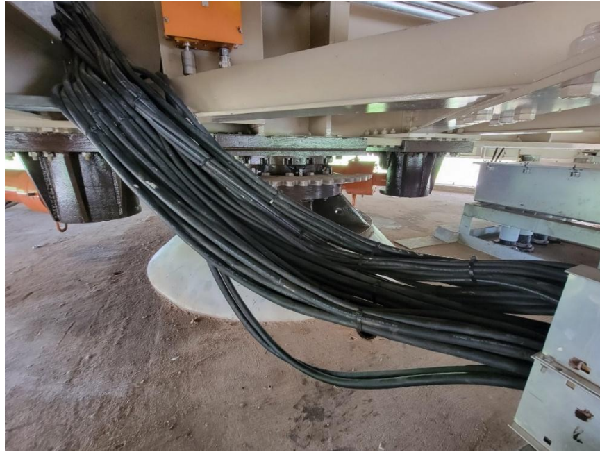
Figure 4-56: Droop cabling used on a swing-span bridge.
