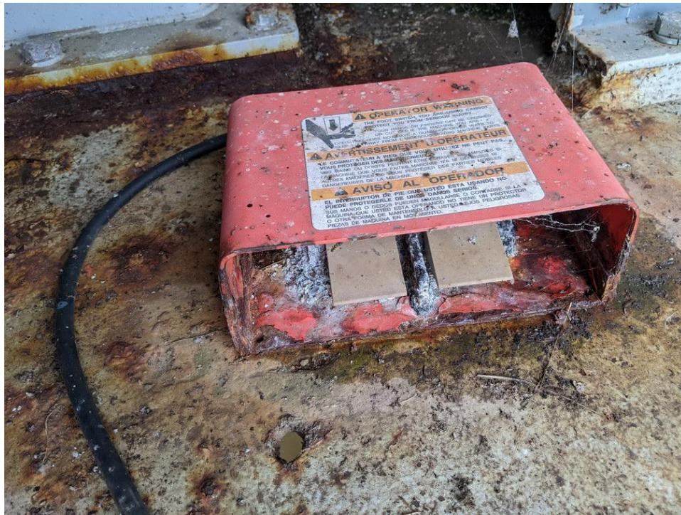
Figure 4-25: Foot switch used for manual control of an auxiliary winch motor on a pontoon bridge. The switch has heavy corrosion with paint failure and dirt/dust debris build-up, rendering the switch is inoperable.
