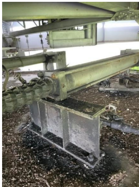
Figure 3-55: A horizontally mounted cylinder on a hydraulically operated swing bridge.
