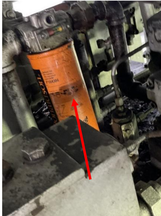
Figure 3-56: Cartridge style filter in place on the primary hydraulic system of a hydraulically operated swing bridge.
