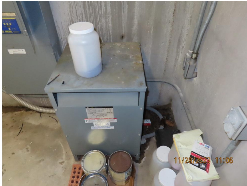
Figure 4-41: Lighting transformer inside an operator house. Articles are stored in front of and on top of the transformer.
