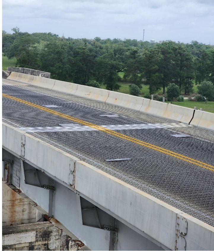
Figure 5-9: Grid deck on bascule bridge with multiple repairs to deck using cover plates.
