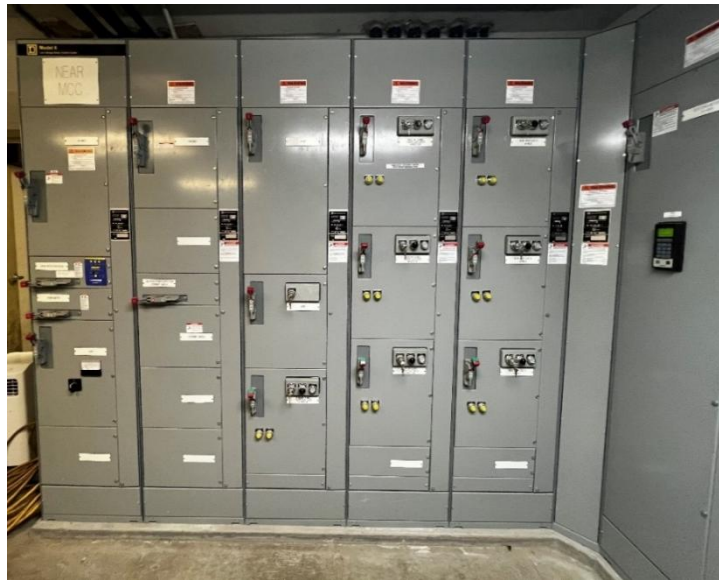
Figure 4-20: Motor control center used for a rolling bascule bridge.
