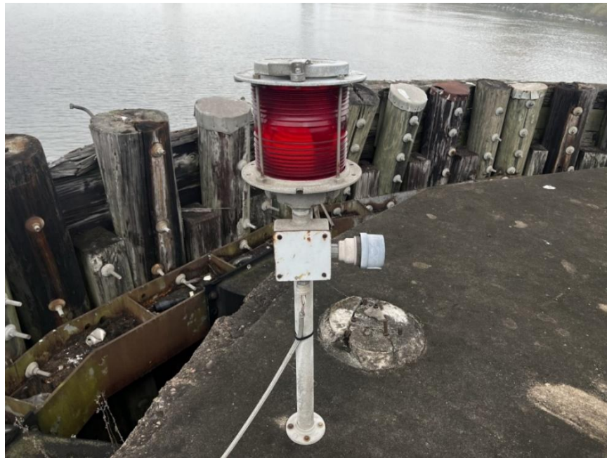
Figure 4-32: Fender navigation light with photocell attached.
