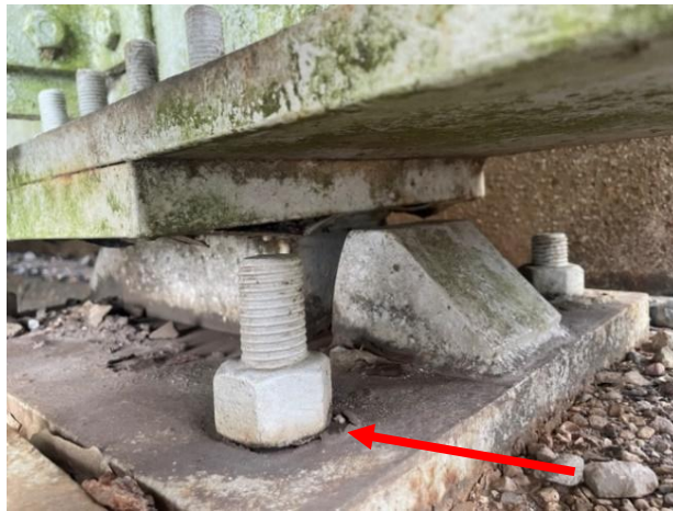
Figure 3-34: Vertical lift centering device. The hardware of the base plate at the corner pictured is not properly tightened. Coded CS3 “poor” due to connection defect.
