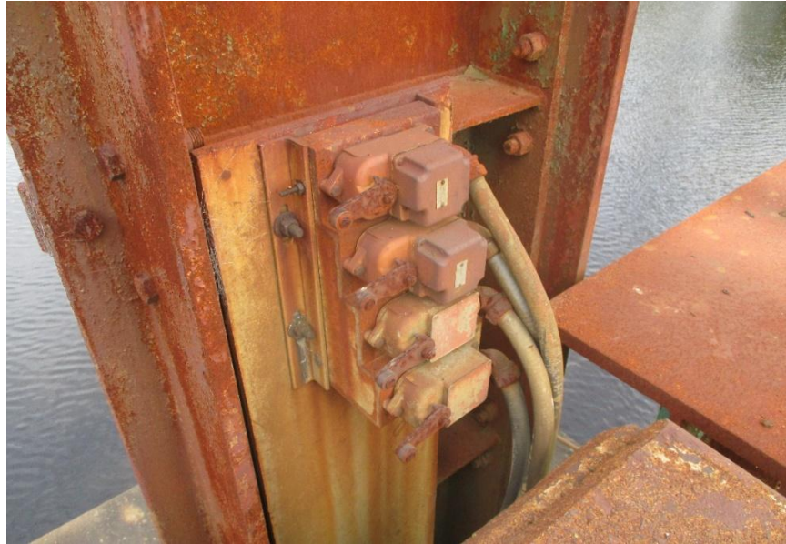
Figure 4-5: Lever arm limit switches used on a vertical lift bridge. Each switch is placed to activate at a different point during opening. Moderate corrosion is present on the entirety of the limit switches.
