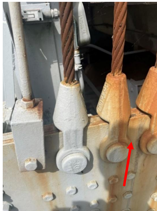
Figure 3-45: Wire rope attachment point to lifting girder of a vertical lift bridge, note corrosion staining.
