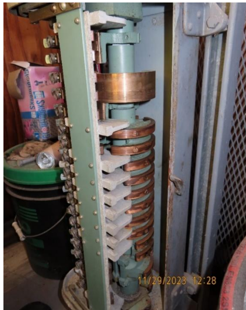
Figure 4-24: Interior of a drum controller.
