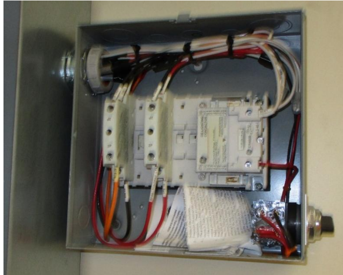
Figure 4-12: Lighting Contactor; note the Auto/Manual Switch on the right side of the box.
