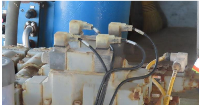
Figure 4-62: Solenoid valves and wiring connections on a control valve block.
