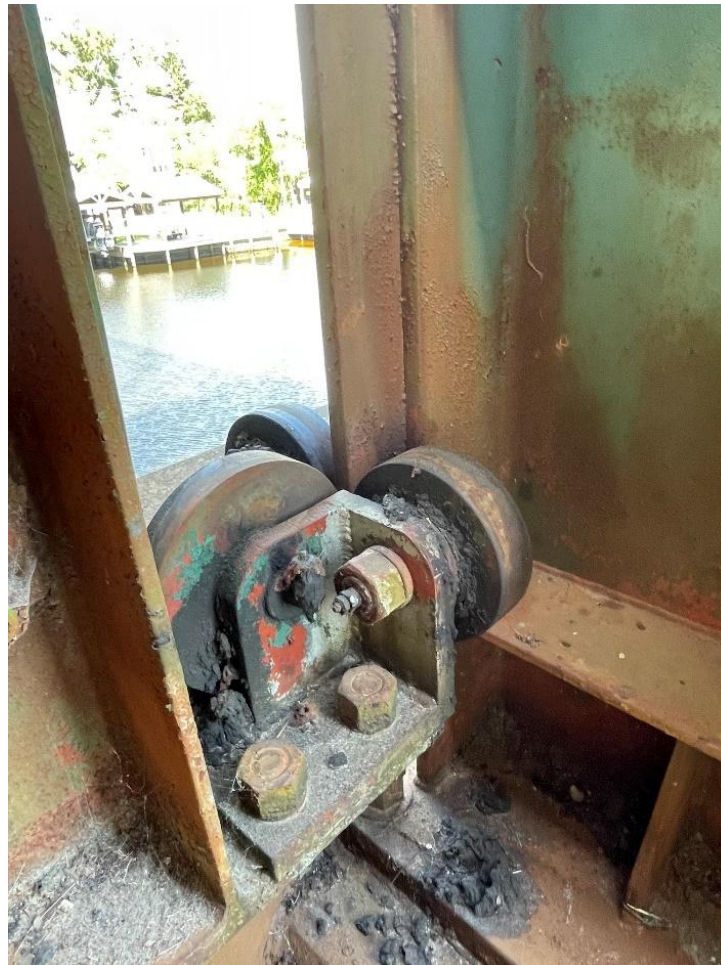
Figure 2-22: Tracks and guide rollers.
