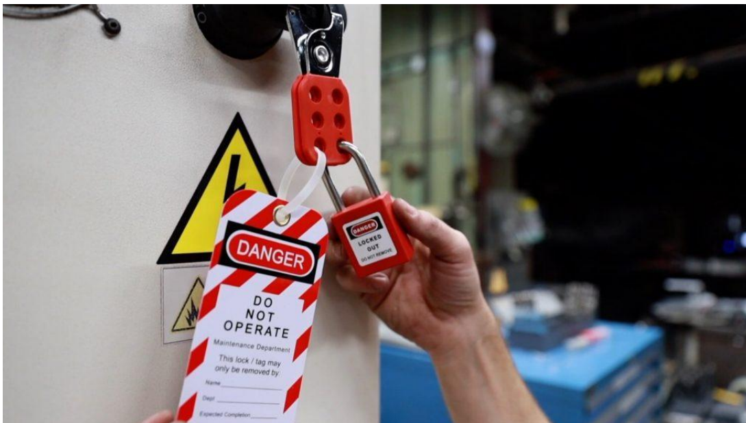
Figure 1-4: Lockout-tagout device on electrical equipment
