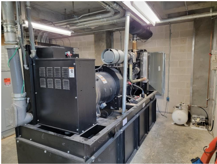
Figure 4-54: Generator inside an operator house.
