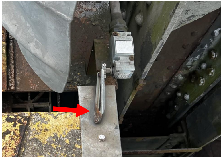
Figure 4-4: Lever arm limit switch. Note that the lever arm is bent, the roller is not making proper contact with the strike plate, and there is rust on the lever arm.
