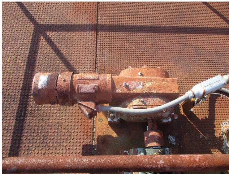
Figure 4-58: Clutch motor used to engage a differential in the gear assembly. Note the heavy corrosion on the motor and clutch assembly.
