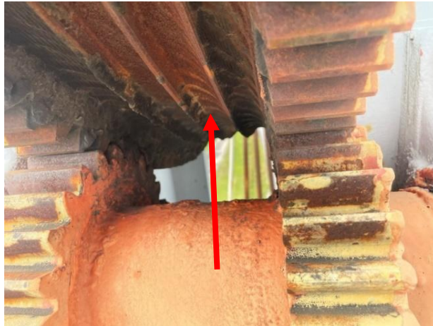
Figure 3-47: Sheave grooves of a vertical lift, with signs of abrasive wear corresponding to the wire rope lay.
