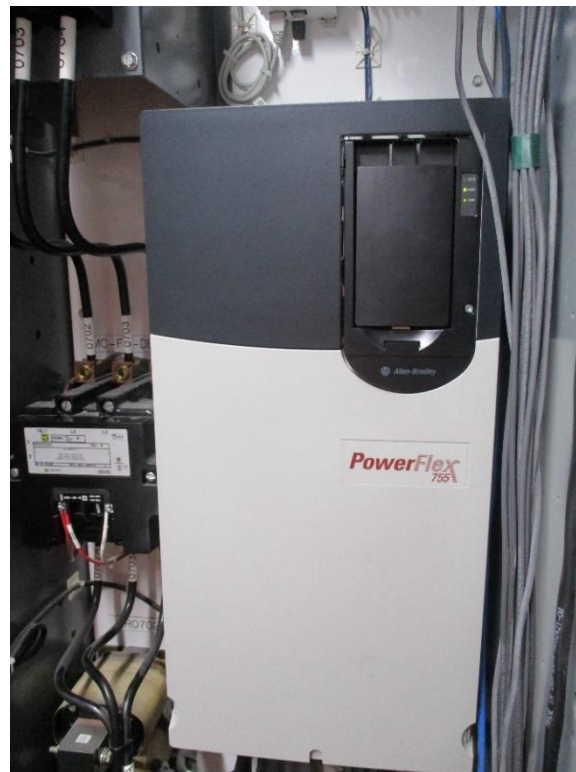
Figure 4-26: Variable frequency drive used to control an AC induction motor, located in an MCC enclosure.
