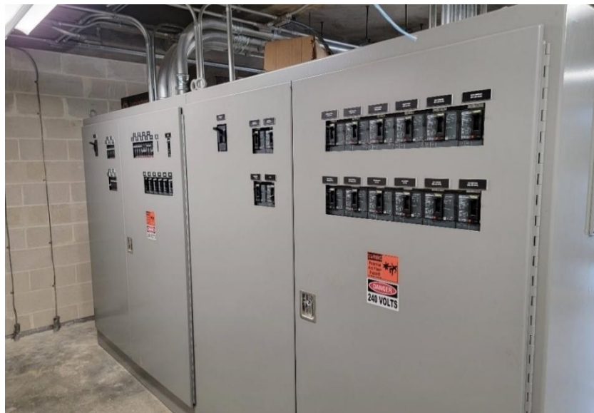
Figure 4-21: Switchboard for a swing-span bridge has warning labels; however, NFPA 70E Arc Flash labels are not present.
