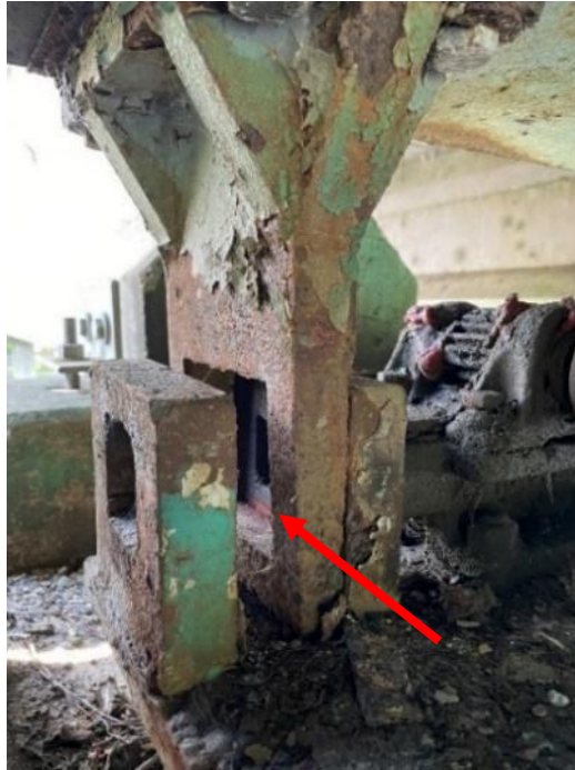
Figure 3-28: Vertical lift span locks inoperable in the released position. Fractured gear tooth. Coded CS3 "poor" due to moderate corrosion defect.
