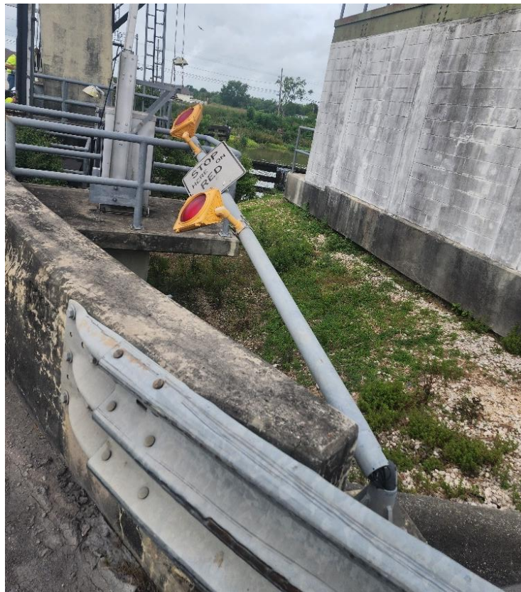
Figure 5-12: Example of broken warning lights and sign.
