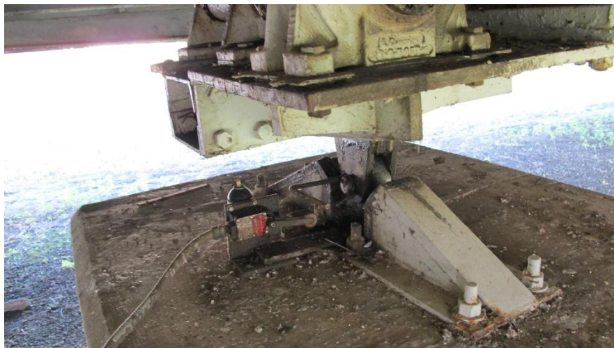
Figure 3-35: Swing-Span centering latch located below the span of a bob-tail swing-span.
