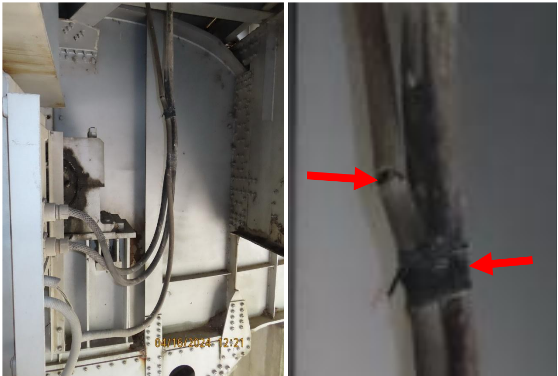
Figure 4-60: Droop cables used on a bascule bridge. Note the cables are cracked, broken, and deteriorating, and the cabling is grouped together using tape (enlarged in photo on the right).
