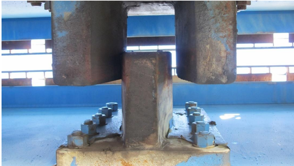
Figure 3-33: Centering device of a double leaf bascule bridge, view is from below the centering device. Note that the centering device is in hard contact on one side. Coded CS3 “poor” due to alignment defect.
