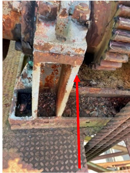
Figure 3-36: Extensive paint failure and corrosion of a vertical lift machinery base. Coded CS4 “severe” due to heavy corrosion defect.
