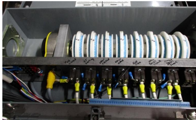
Figure 4-9: Rotary cam limit switch inside enclosure. No notable deficiencies.
