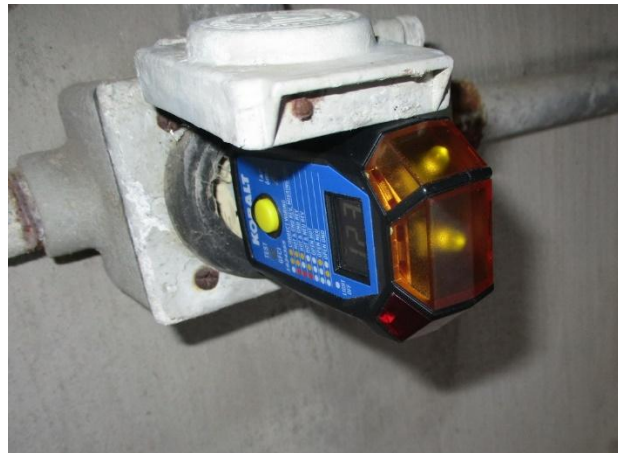
Figure 4-1: GFCI receptacle tester plugged into a receptacle. The two yellow lights on the tester are illuminated while the bottom light is not, indicating the receptacle is functioning- energized and correctly wired.
