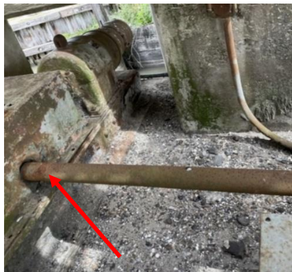
Figure 3-5: Paint failure and corrosion of a machinery shaft, should be coded CS3 “poor” due to moderate corrosion defect.
