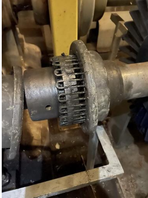
Figure 3-10: Grid coupling with a sleeve half removed for internal inspection, coupling coded CS3 “poor” due to inadequate lubrication.
