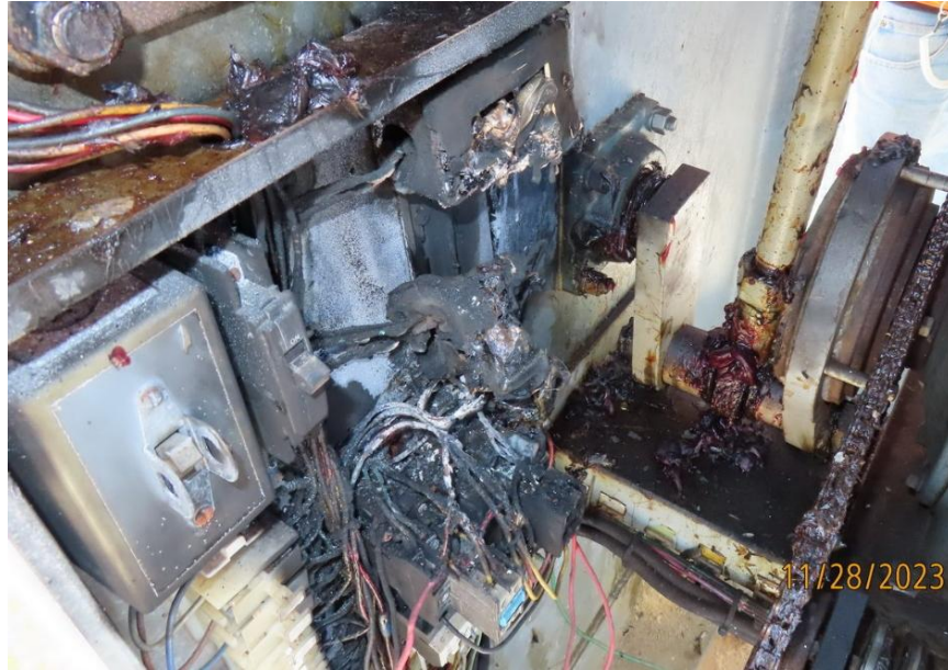
Figure 1-2: Evidence of a fire inside a traffic barrier gate, note the scorch marks and melted components.
