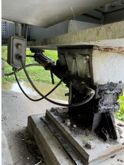
Figure 3-43: Live load support of a swing bridge. The element pictured is outboard of the balance wheels on the center pivot pier and utilizes a hydraulic operated wedge.
