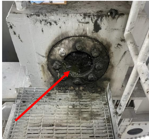
Figure 3-4: Excessive contaminated lubricant of the trunnion bearing of a bascule bridge. Coded CS3 “poor,” due to lubrication defect as the lubricants exhibit moderate contamination.
