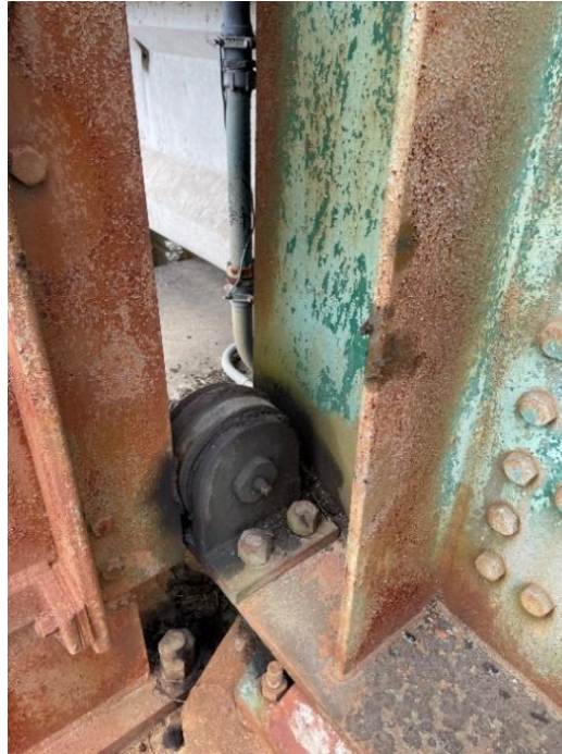
Figure 3-49: Vertical lift span guide angle and roller.
