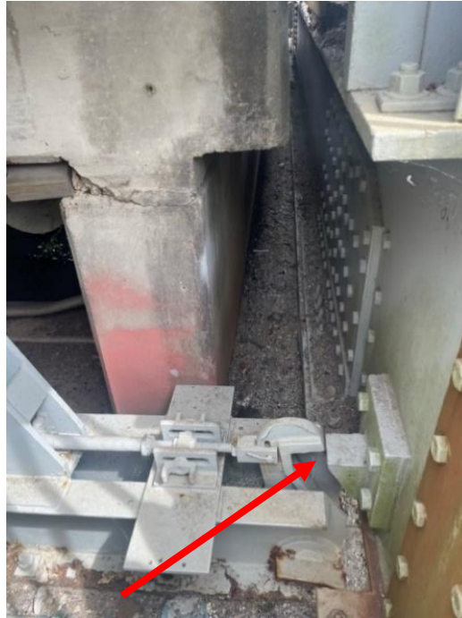
Figure 3-29: Latch style vertical lift span locks, inoperable in the open position. Coded CS4 “severe” due to operational defect.
