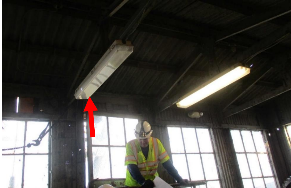
Figure 4-35: Fluorescent fixtures in a machinery room. Note that one of them is not functioning.
