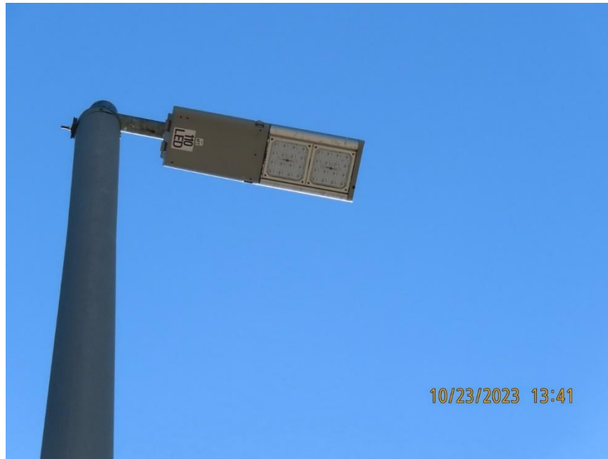
Figure 4-34: LED roadway luminaire.
