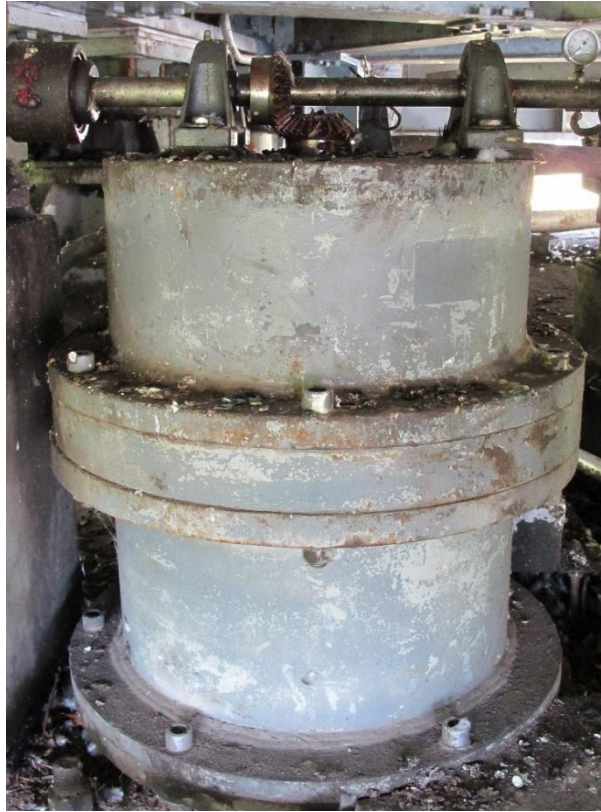
Figure 3-41: Drum differential of a swing bridge. Drum differential coded CS2 "fair" due to minor corrosion defect.
