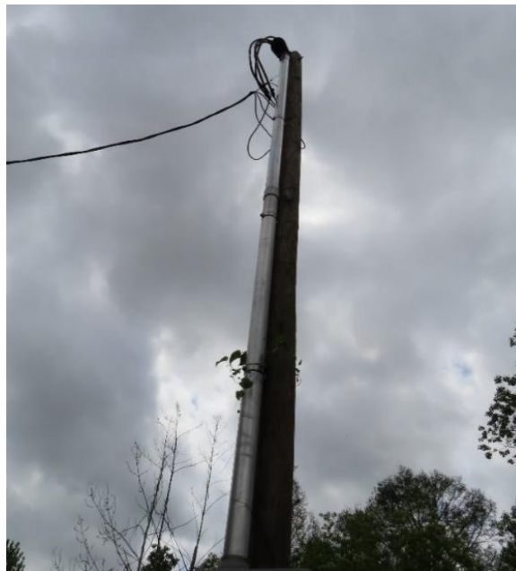
Figure 4-37: Weather head and cable drip loop for utility service.
