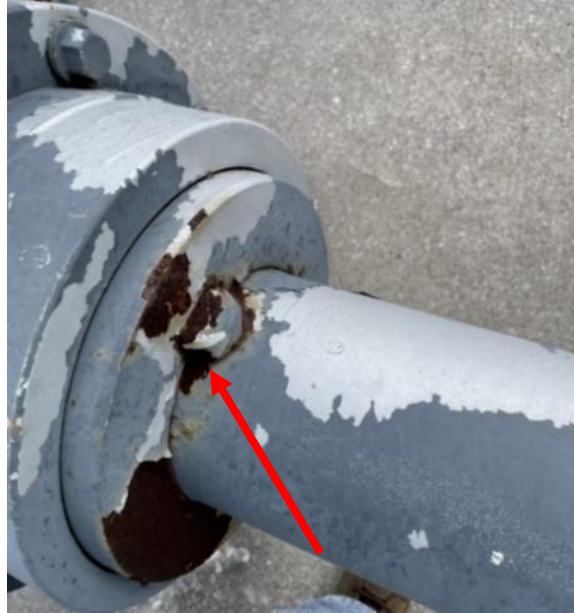
Figure 3-6: Corrosion and paint failure at intersection of shaft keyway shoulder and key. Shaft coded CS3 “poor” due to moderate corrosion defect.
