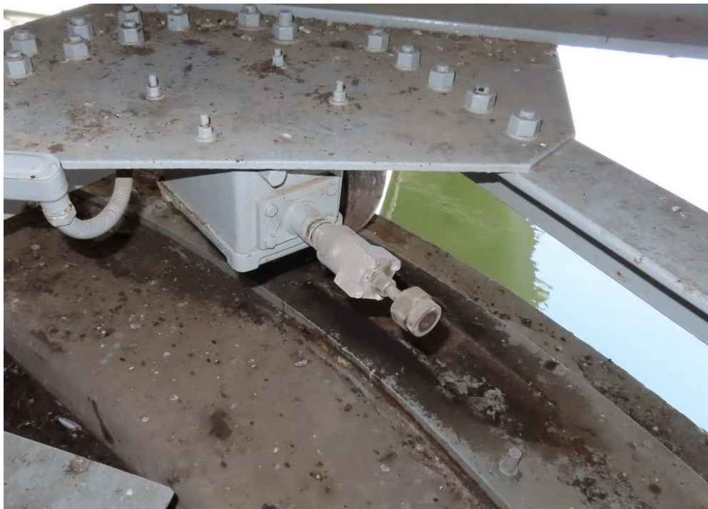
Figure 4-6: Plunger limit switch on a swing-span bridge. Note the dirt and dust buildup.
