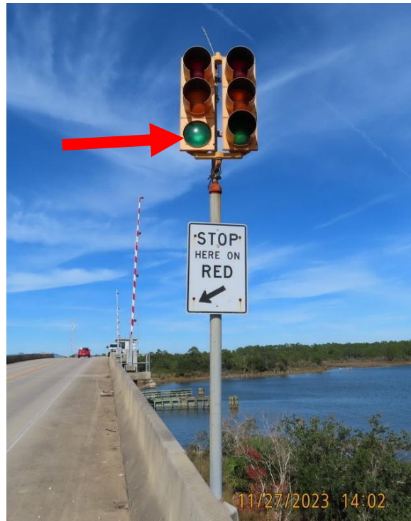
Figure 4-31: Tri-color traffic signals. Note the missing visor on the left green light.
