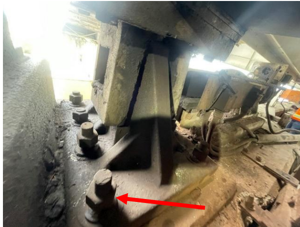
Figure 3-30: Live load shoes of a bascule bridge, designed to accept a lock bar. The hardware of this live load shoe base is not properly tightened. Coded CS3 "poor" due to connection defect.
