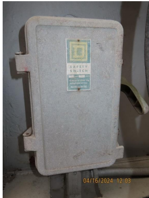
Figure 4-49: Disconnect switch used for a motor. Note the lack of labeling indicating what motor it's for and no arc flash labeling.
