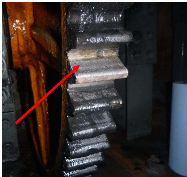
Figure 3-21: Abrasive wear of open gearing. Coded CS3 “poor” due to damage defect.
