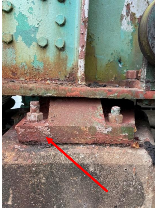
Figure 3-31: Live load shoe of a vertical lift bridge. Coded CS4 “severe” due to heavy corrosion.
