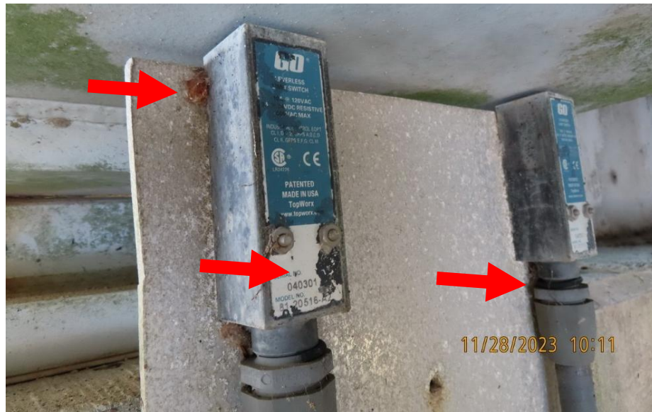
Figure 4-7: Two proximity limit switches on a bascule bridge. Note the minor rust around the mounting plate for the switch, the label is deteriorating, and the conduit connection is loose.
