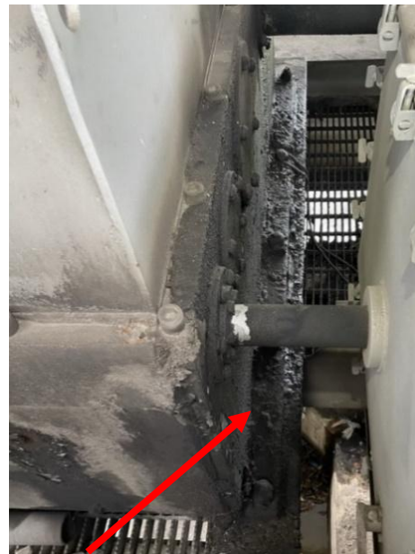
Figure 3-13: Evidence of oil leaking past seals in a primary reducer, should be coded CS3 “poor” due to lubrication defect.
