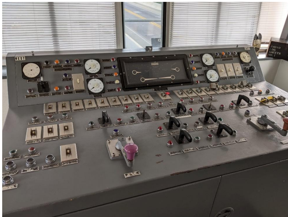
Figure 4-16: Control desk inside of an operator house on a bascule bridge. No notable deficiencies. Note that the dials used to relay information about the bridge are old, and personnel should verify that the dials are functional during operation, as equipment of that age tends to fail over time.
