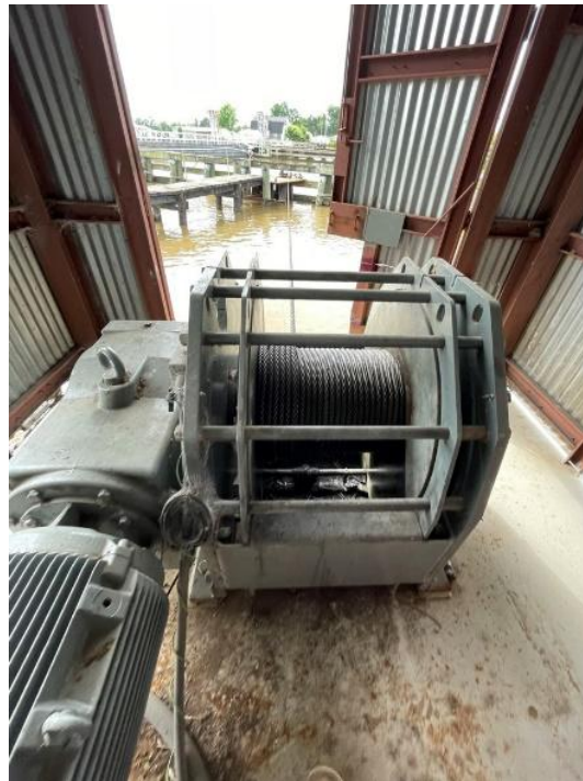
Figure 2-37: Electric operational winch of a pontoon bridge.
