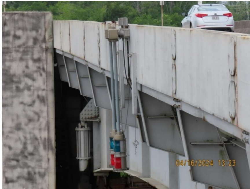
Figure 4-33: Span navigation lights on a bascule bridge.
