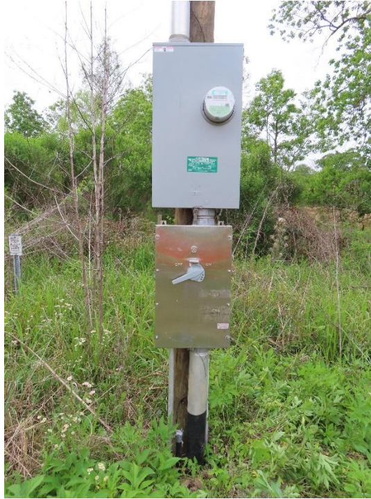
Figure 4-38: Service disconnect switch and service meter.
