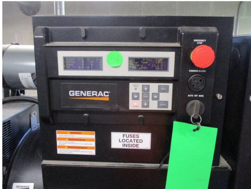
Figure 4-55: Generator control panel.
