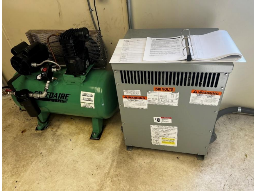
Figure 4-40: Lighting transformer inside an operator house. Articles are on top of the transformer.
