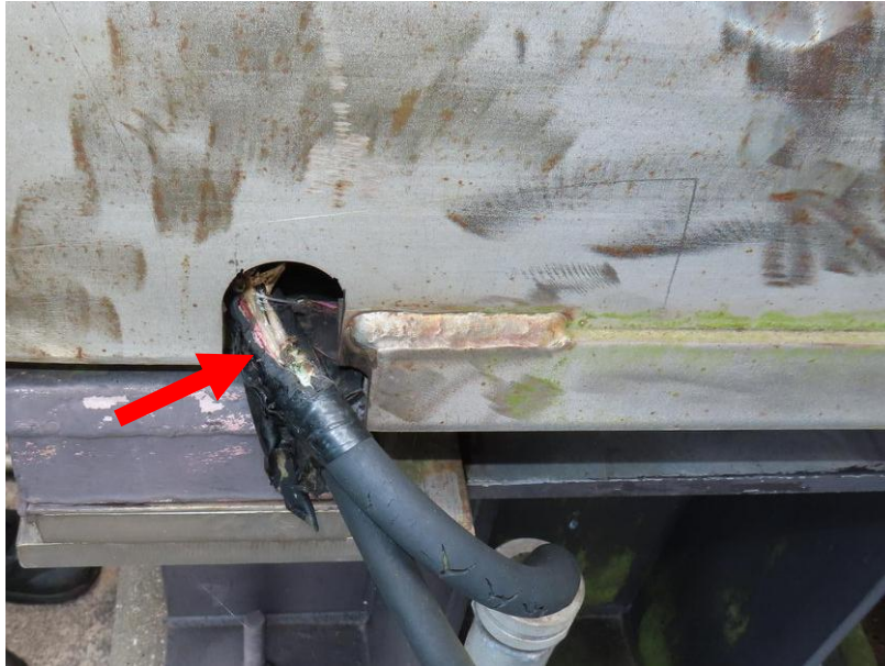
Figure 4-42: Damaged flexible cable jacket with interior wiring showing.
