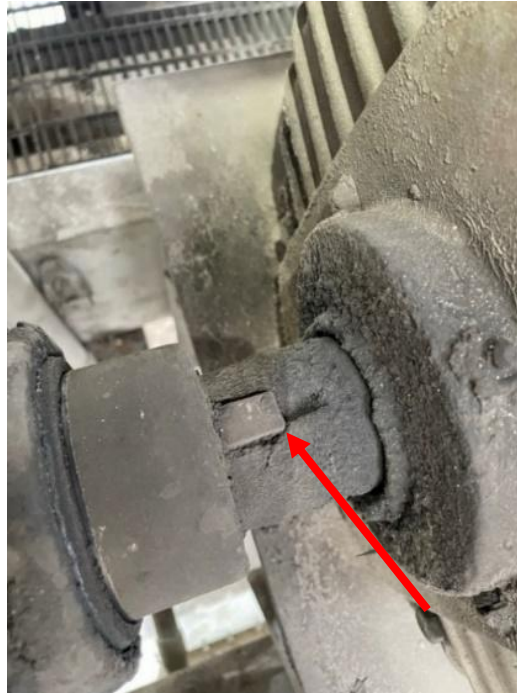
Figure 3-38: Key and keyway of a bascule bridge drive shaft. Note excess grease, and contamination of area, and possible fatigue crack of the shaft.
