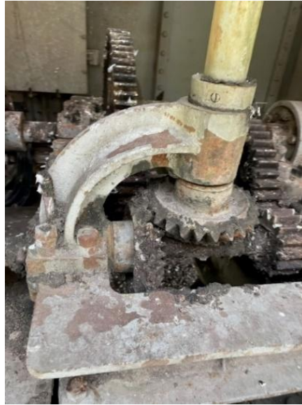
Figure 3-19: Bevel gears of a swing bridge.
