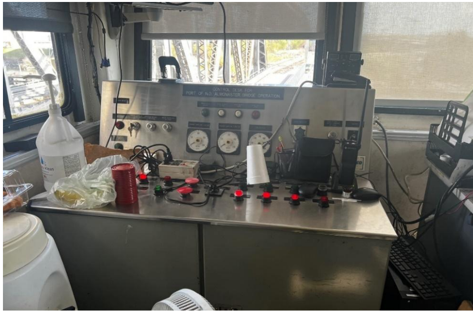
Figure 4-15: Control desk inside of an operator's house used on a Strauss-trunnion bridge. Note the excessive clutter on the desk, cups are used to cover up buttons, and some lights and switches are obscured by loose articles.
