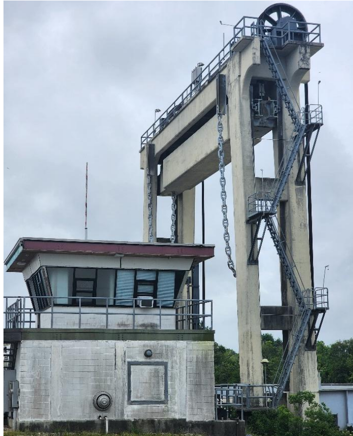
Figure 5-4: Vertical lift bridge with concrete towers supporting bridge machinery, sheaves, and lifting cables.
