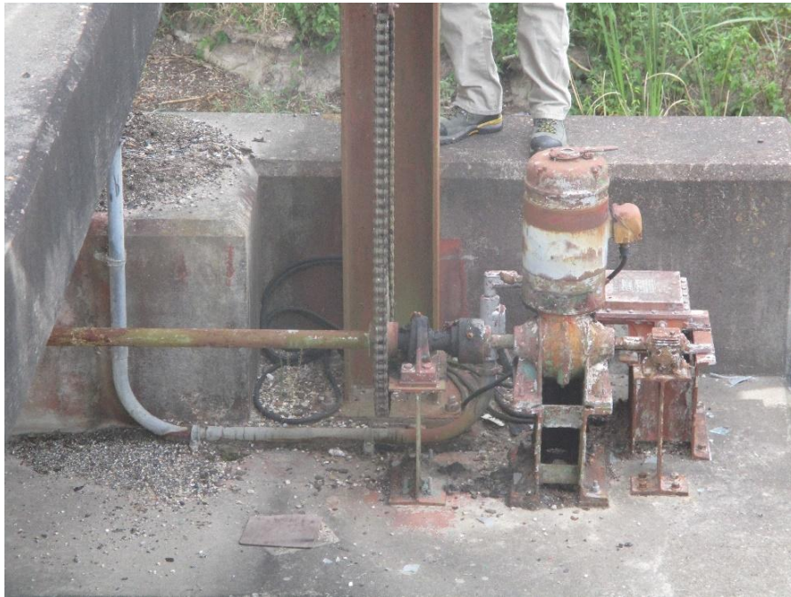
Figure 4-30: Machinery for a traffic barrier. The equipment has been painted, but areas with moderate corrosion remain (not clearly visible in this photo).
