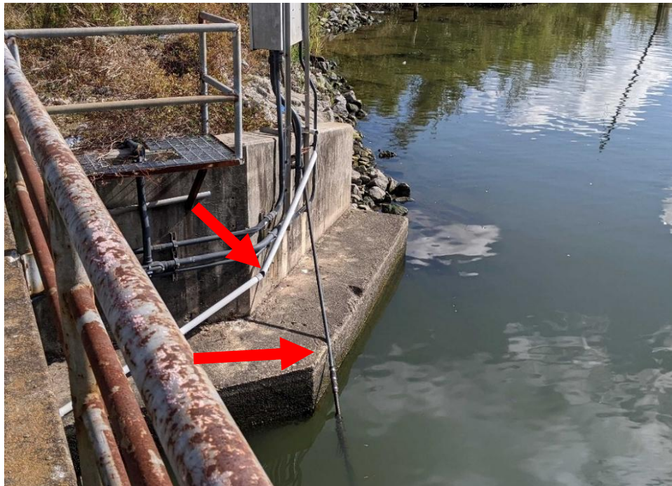
Figure 4-46: Submarine cable entering a channel. The submarine cable is under tension, insufficiently supported, and subject to abrasion on the concrete. In addition, conduits are broken around the area.
