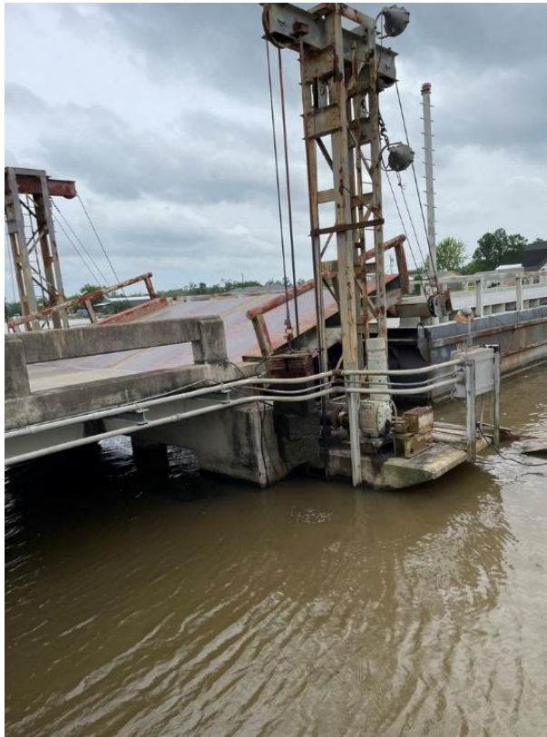
Figure 2-39: Pontoon bridge apron ramp and machinery towers during operation.
