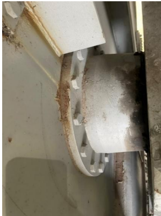
Figure 3-53: Trunnion of a bascule bridge, bolted to the trunnion girder.
