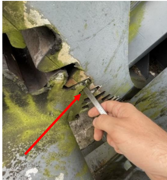
Figure 3-16: Measurement of gear backlash in the field with a taper gauge.
