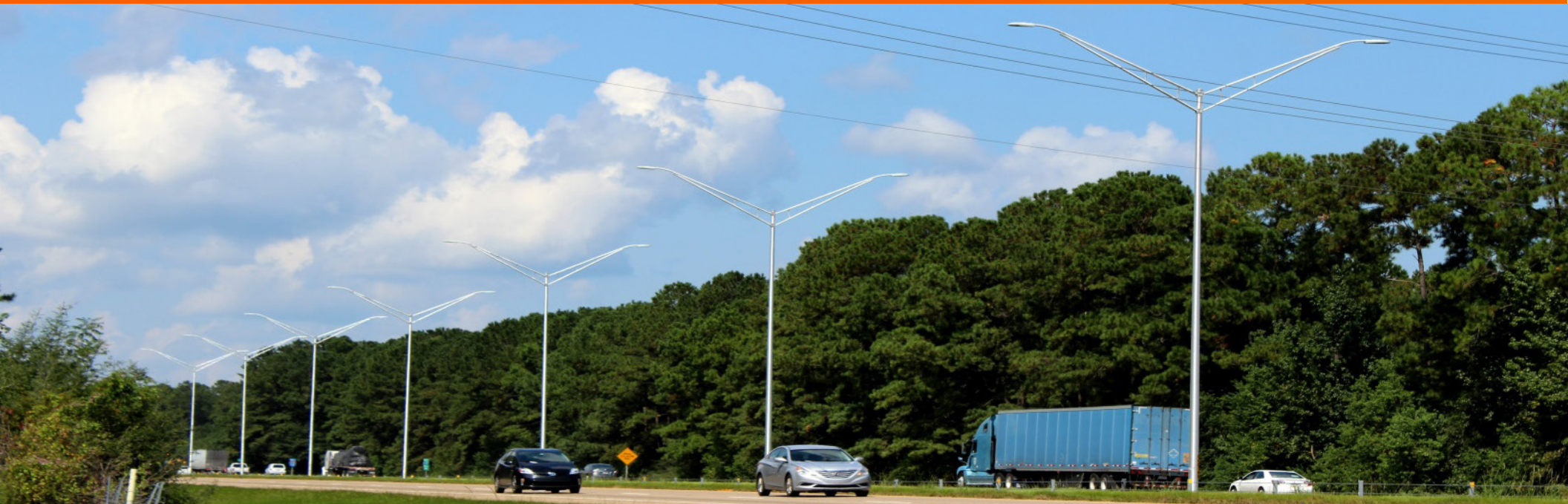
GEC-DESIGNED LIGHTING ALONG I-12
