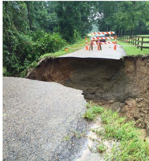
Figure 1: Flooding Damage of Old Tunica Road in St. Francisville
