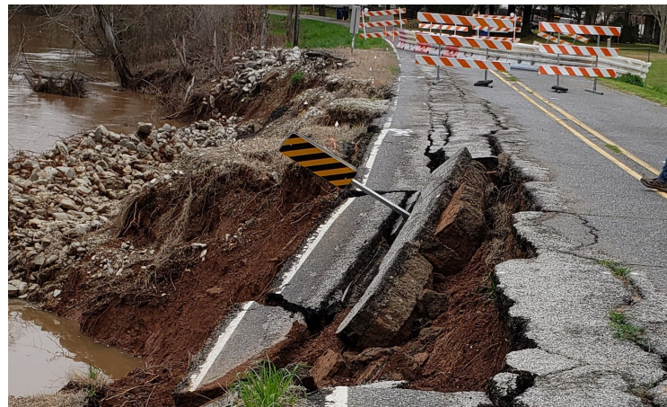
Slope failure along LA 745
