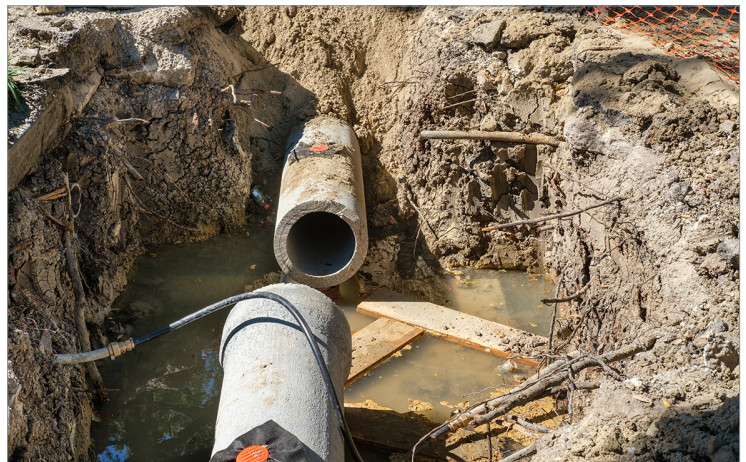
Damaged pipes and standing water in an open hole during street repairs in New Orleans
