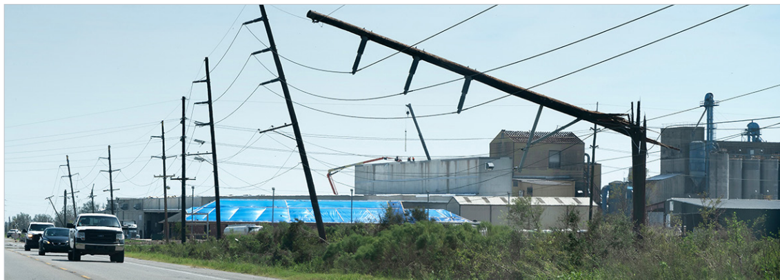
September 6, 2020: Damage from Hurricane Laura in Lake Charles, Louisiana
