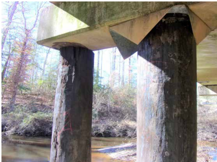
Timber piles needing to be shifted on LA 348
