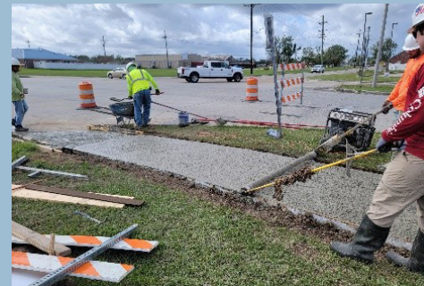
Figure 2. Our team provides consistent on-site presence throughout all phases, enabling real-time quality assurance and swift resolution of construction challenges.
