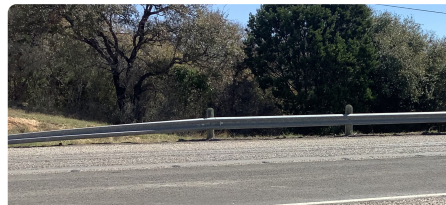
H&H field crew confirmed existing guardrail, transition to bridge rail, and end down turn were not MASH compliant on Hazard Elimination and Safety Improvements project
